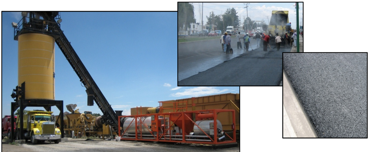
Phoenix Industries, AR150M asphalt rubber blending plant at Mezcla Asfáltica de Alta Calidad hot plant site in Toluca, Mexico
